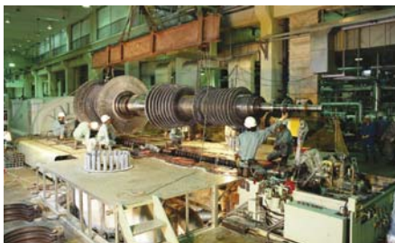
Staff from Okinawa Plant Kogyo Company, Limited disassemble a turbine at Makiminato Thermal Power Plant for a regular inspection.
