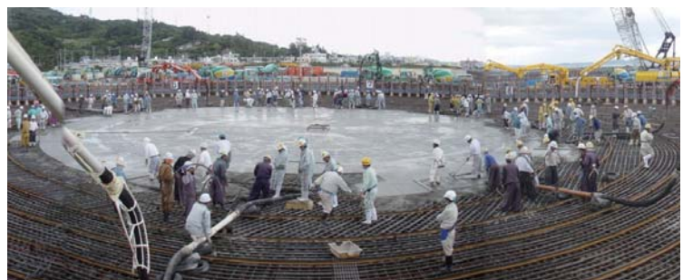
Pouring the concrete foundations for the No.1 LNG tank at the Yoshinoura thermal power plant
