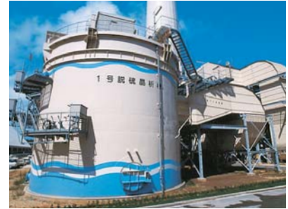
Environmental protection facilities at a power plant
