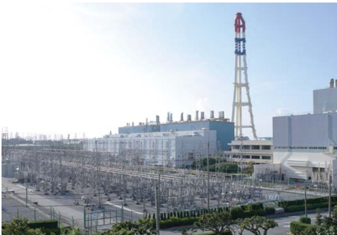
Makiminato thermal power station
