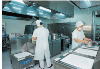
Welfare facility with an all-electric kitchen
