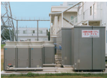
Ice-storage air conditioning systems
