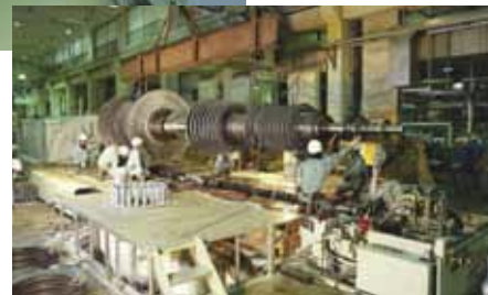
Staff from Okinawa Plant Kogyo Company, Incorporated disassemble a turbine at Makiminato Thermal Power Plant for a regular inspection.
