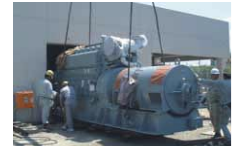
Employees of Progressive Energy Corporation (PEC) install a small-scale power generator, part of a "distributed generation" network.
