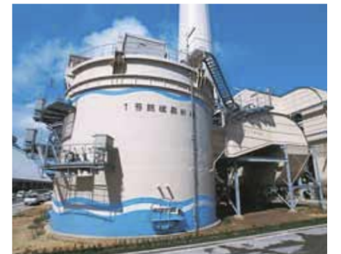
Environmental protection facilities at a power plant As part of an overall policy of removing harmful chemicals from smoke emitted by our power plants, they are equipped with desulphurization and denitrification equipment.
