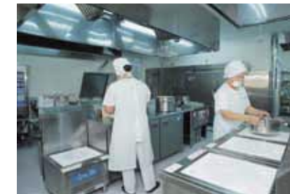
Welfare facility with an all-electric kitchen
