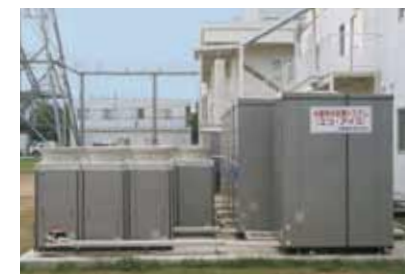
Ice-storage air conditioning systems
