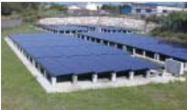
Field tests on an industrial solar power system are being carried out at a facility on Kita-Daito Island.
