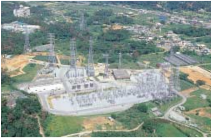
The transformation facility in Enobi
